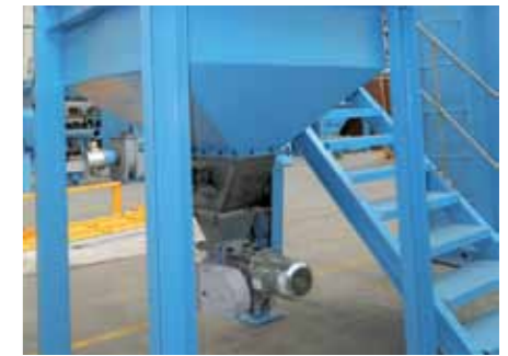
Lime dosing units
